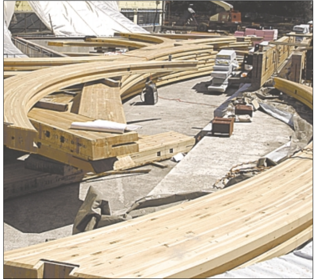
These wood 'glulams' were put together like a jigsaw puzzle to create the hospital's new main lobby and to adorn the cancer centre waiting areas.
