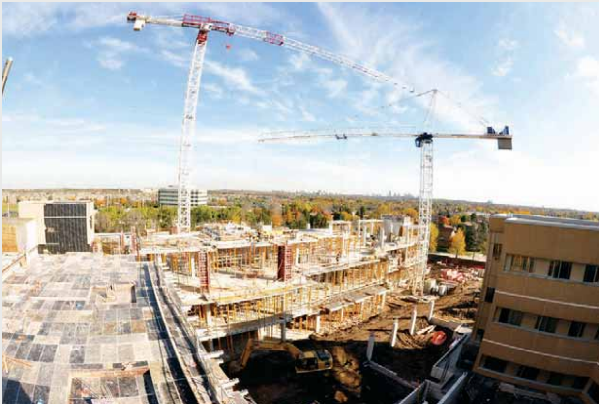
ABOVE: Substantial progress has been made. The footings and foundations were in place July 2008. The exterior wall framing and sheathing will be completed by January 2009. Construction crews are currently working on level 3, and they are working diligently to complete the structure before the snow falls. We'll "top off" the A wing structure in December, which means the building will be enclosed soon afterward.
